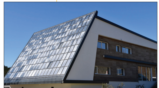
▲ Figure 9. Collectors used for hot water preparation and air heating at the T&T Headquarters (Project Senergy Force) in Vouzela, Viseu, Portugal
