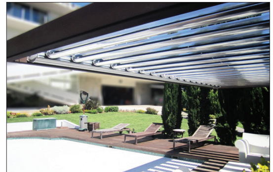
▲ Figure 8. Collector used for swimming pool heating in Estoril
