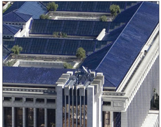
▲ Figure 4. Solar thermal installation at the CGD's Headquarters in Lisbon, Portugal
