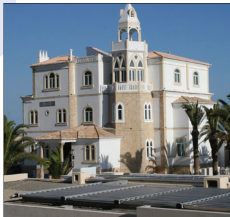
◀ Figure 7. Collectors used for hot water preparation and swimming pool heating at the Bela Vista Hotel and Spa in Paria da Rocha
