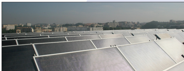
▲ Figure 6. A solar thermal installation with flat plate collectors produced by the Portuguese company OpenPlus for domestic hot water preparation (580 m 2 ) in Matosinhos, Portugal (photo credit: Openplus)
