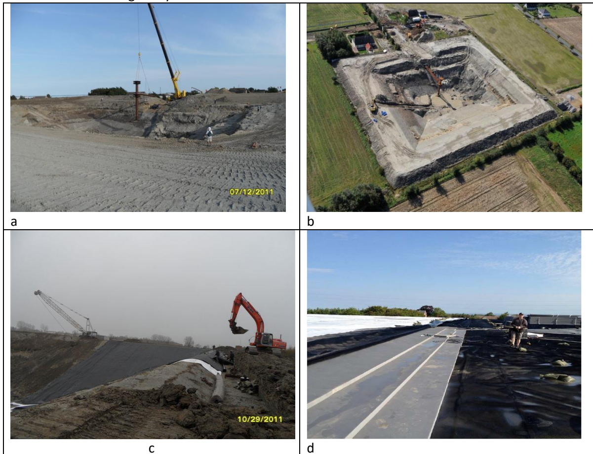
Figure 20 Construction of the storage in Marstal [13]. a: inlet and outlet pipes are hoisted into place. b: the storage after the cloudburst. c: The liner work. d: the lid is built.
