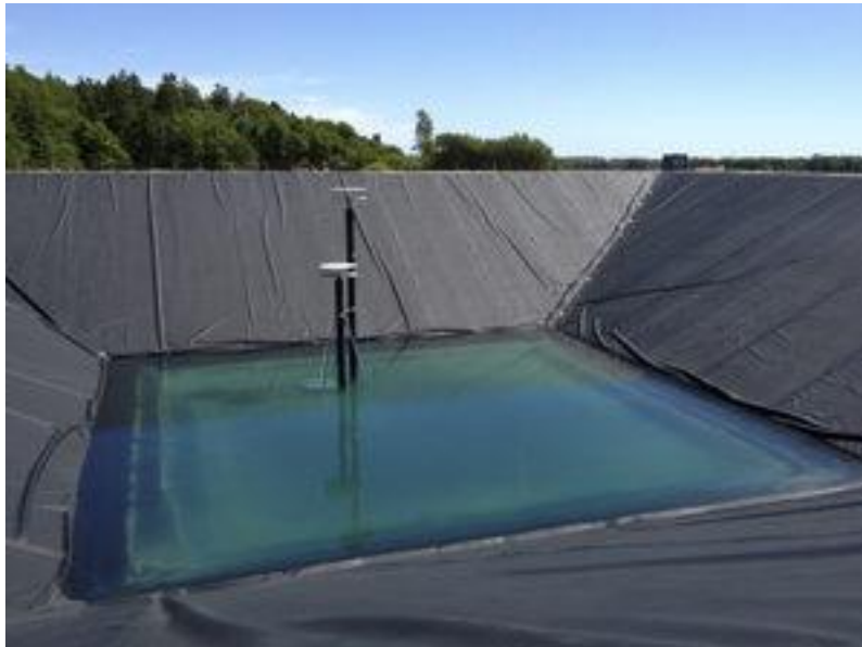
Figure 1. Picture of Dronninglund Pit Storage under construction. Dronninglund District heating; 37,573 m 2 of solar collectors and a 60,000 m 3 water in pit heat storage. (PlanEnergi)
