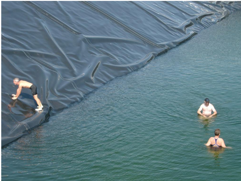
Figure 16 The folds are inspected under the water filling [10].
