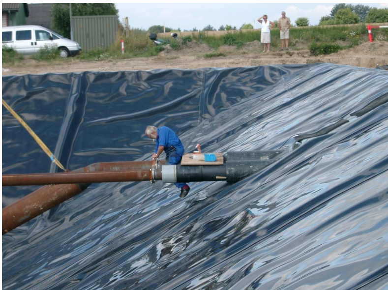
Figure 17 Inlet and outlet pipes. The leak was in the liner weld during one of the pipes [10].
