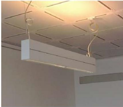
Figure 3. Luminaire with direct and indirect light output.
