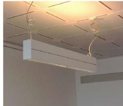
Figure 3. Luminaire with direct and indirect light output.
