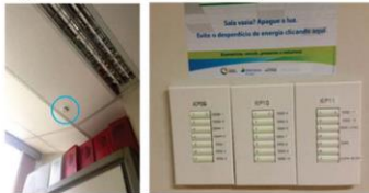
Figure 3. Photosensors close to windows and lighting switch interfaces in corridor.
