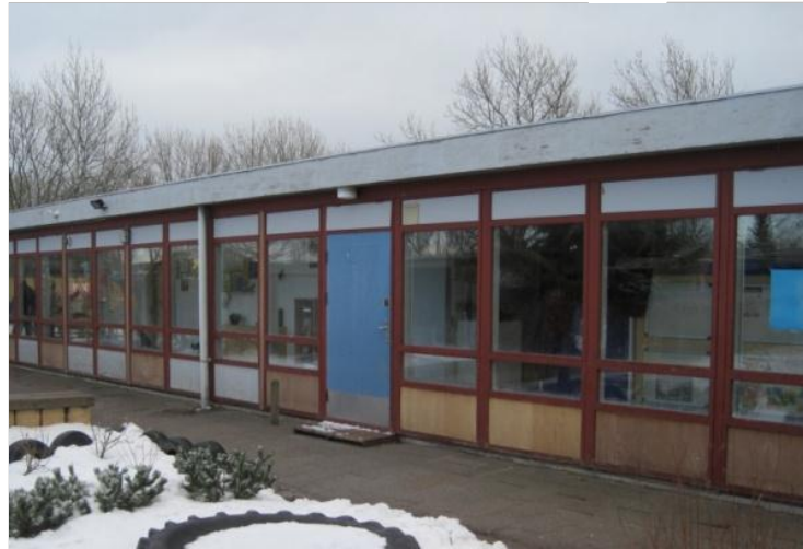
Left: Facade facing the playground before renovation. The painted facade required regular maintenance.
