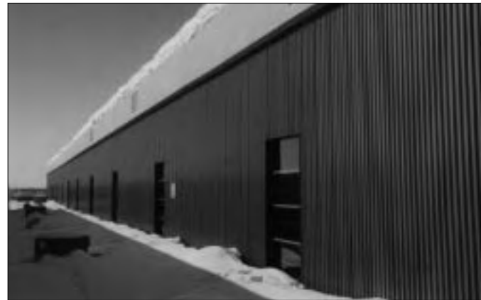
Figure 5: The 10,000 m 2 unglazed solar wall of Bombardier's Canadair aircraft factory in Valcourt, Canada.
